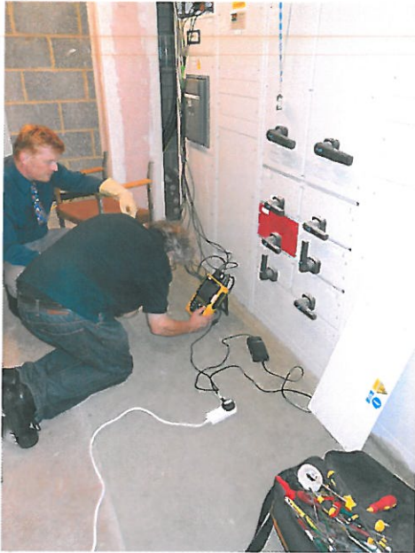
Figure 1- BSRIA's installation of the metering unit used for the trial at the LV Switchboard.
